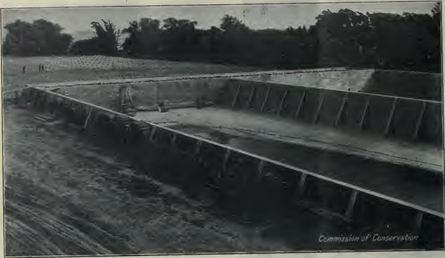
Hamilton Sewage Disposal Works—Tanks and Filtering Beds.
